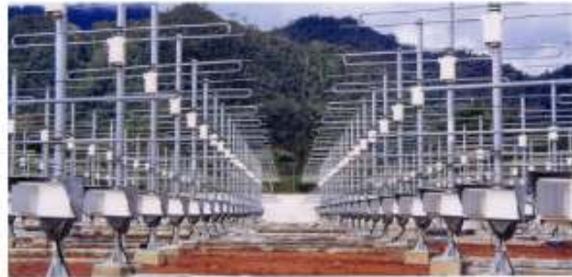
3 elements Yagi antennas
