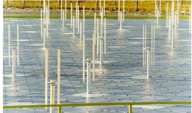
Fig : 6. Reception Antennas
