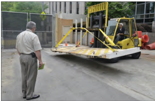
Figure 9: Security improvements at Main State. DS constantly updates and improves security at all U.S. diplomatic facilities. In this image, a DS Security Technical Specialist (left) and a DS contractor remove a vehicle barrier plate in order to lay experimental surface treatment at the Department of State's Harry S Truman building in Washington, D.C. Source: Private collection.
