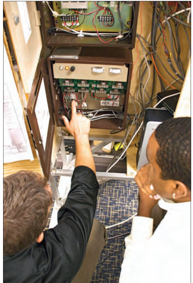
Figure 20: DS Security Technical Specialists, of the Project Management and Engineering branch, troubleshoot a defective door control power supply on a Security Management Systems enterprise test fixture in September 2009. Source: Bureau of Diplomatic Security Files.
