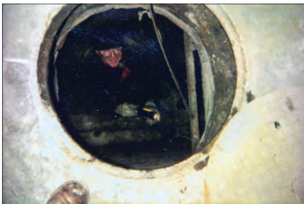
Figure 6: Winter 1994: A DS Security Engineering Officer works to install alarms in the utility tunnels beneath a U.S. embassy overseas. The alarm system was a precautionary countermeasure aimed at alerting embassy security personnel if intruders entered the tunnels. Running beneath public streets, such tunnels sometimes were used in espionage efforts by foreign intelligence operatives. Source: Private collection.
