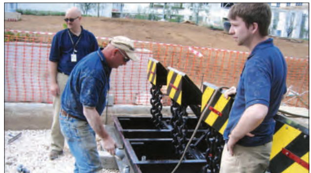
Figure 20: A U.S. Navy Seabee Building Chief Petty Officer, a DS contractor, and a Senior DS Engineer (left to right) replace a Delta Barrier in Athens, Greece, in 2008. After the Al-Khobar Towers bombing, DS obtained additional resources to improve security at U.S. posts overseas. DS also became an active member of the Counterterrorism Subcommittee of the National Security Council. Source: Bureau of Diplomatic Security Files.
